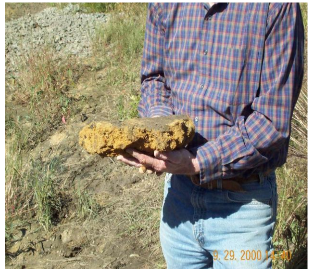
Soil in this basin has been compacted due to improper construction methods that led to this basin retaining water and causing subsequent compaction from the sheer weight of the water column.
